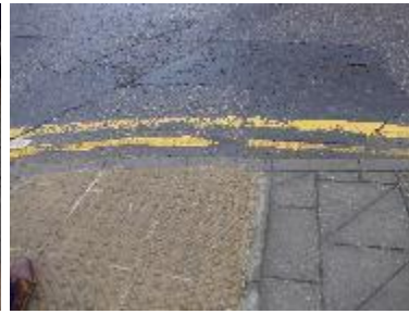
Barclay St tactile paving
